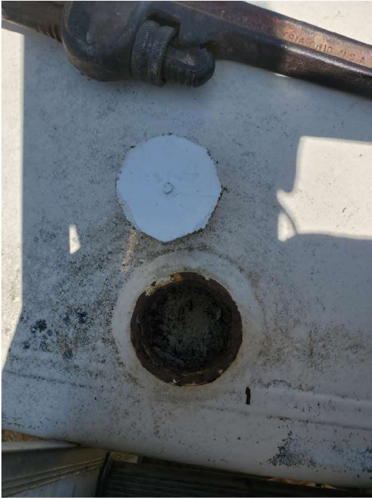
Photo 6. Secondary containment and interstitial space insulation
