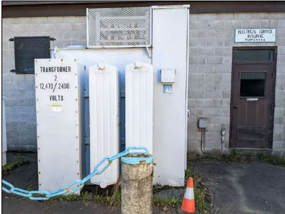
Transformers 2 and 2a
