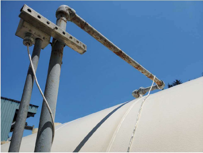
Photo 8. Dispensing piping and liquid level gauge
