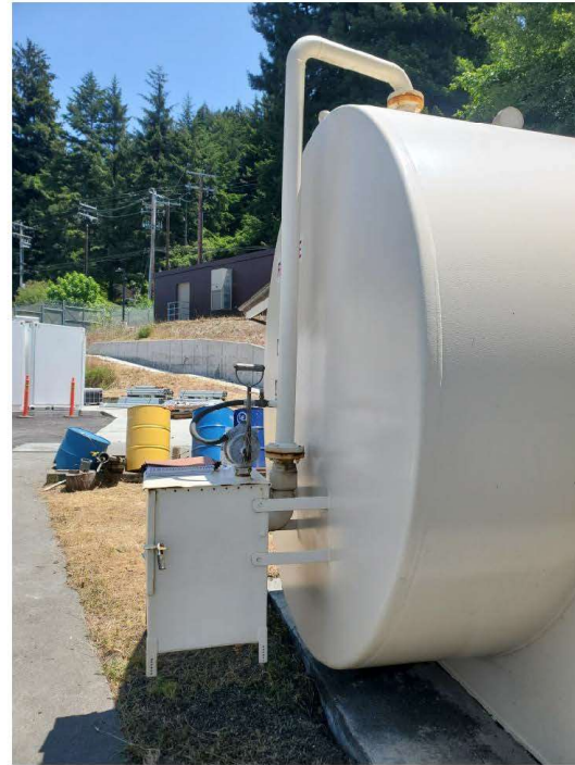
Photo 7. Fill piping and spill box
