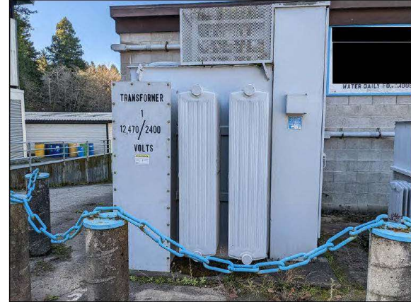
Transformers 1 and 1a
