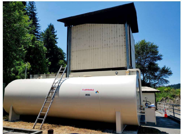
Photo 1. AST-1: 10,000-gallon double-walled diesel steel tank
