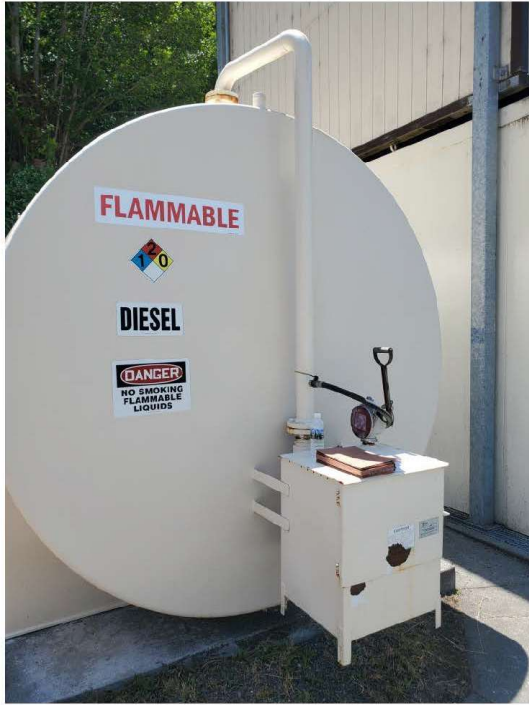
Photo 2. AST-1: 10,000-gallon double-walled diesel steel tank
