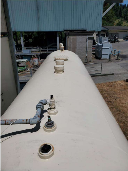
Photo 12. Emergency vents and liquid level gauge
