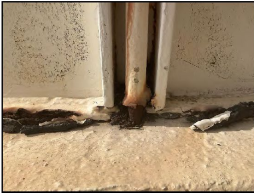
033 Active Corrosion on Anchor Chair Z
