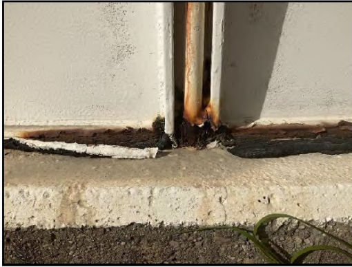
031 Active Corrosion on Anchor Chair X
