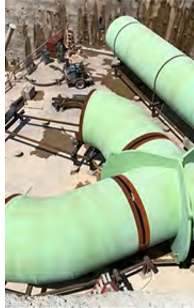
Steel Water Pipe Section
