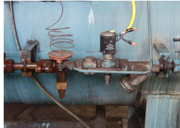
Exposed electrical wiring
