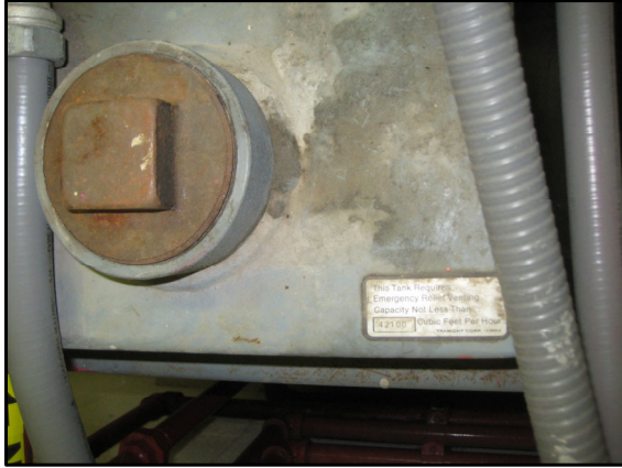
Steel plug on emergency vent on day tank
