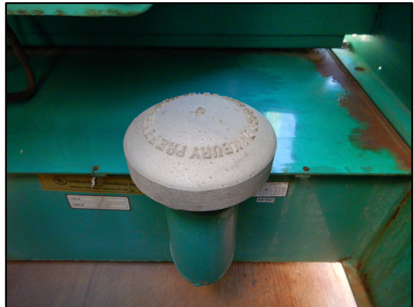
Rated emergency vents not installed, nor properly terminating above grade outside of the enclosure
