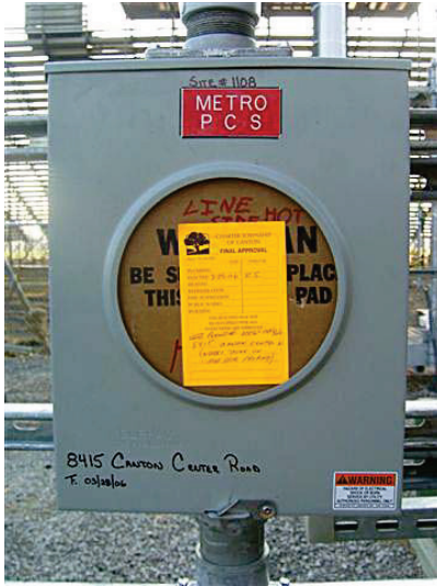
Figure 2-3 Example of an inspected and approved installation ready to be connected to the utility's power grid. Source: Trinity Technologies http://www.trinitytechelectric.com/images/cell/Electrical/Final%20inspection%20sticker%20(3).jpg .
