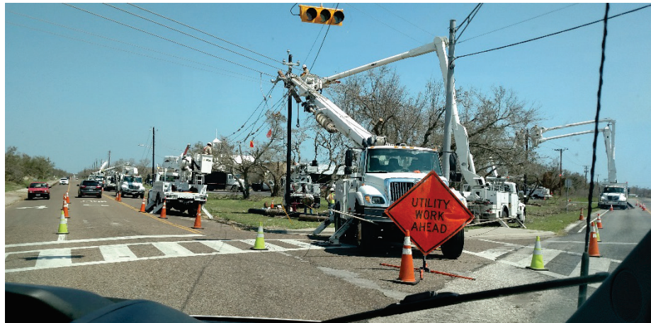
Figure 2-2 Power restoration after Hurricane Harvey.
