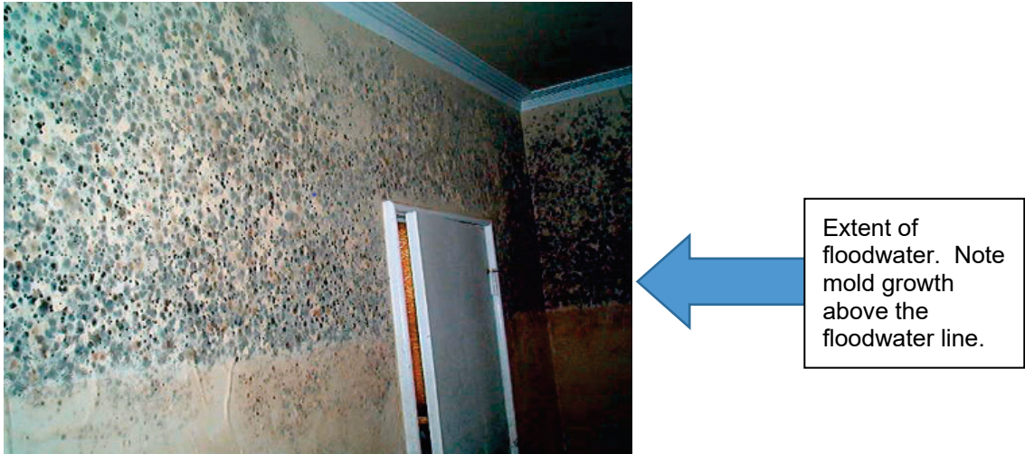
Figure 4-2 Look for mold growth above the floodwater level (FEMA, 2006).
