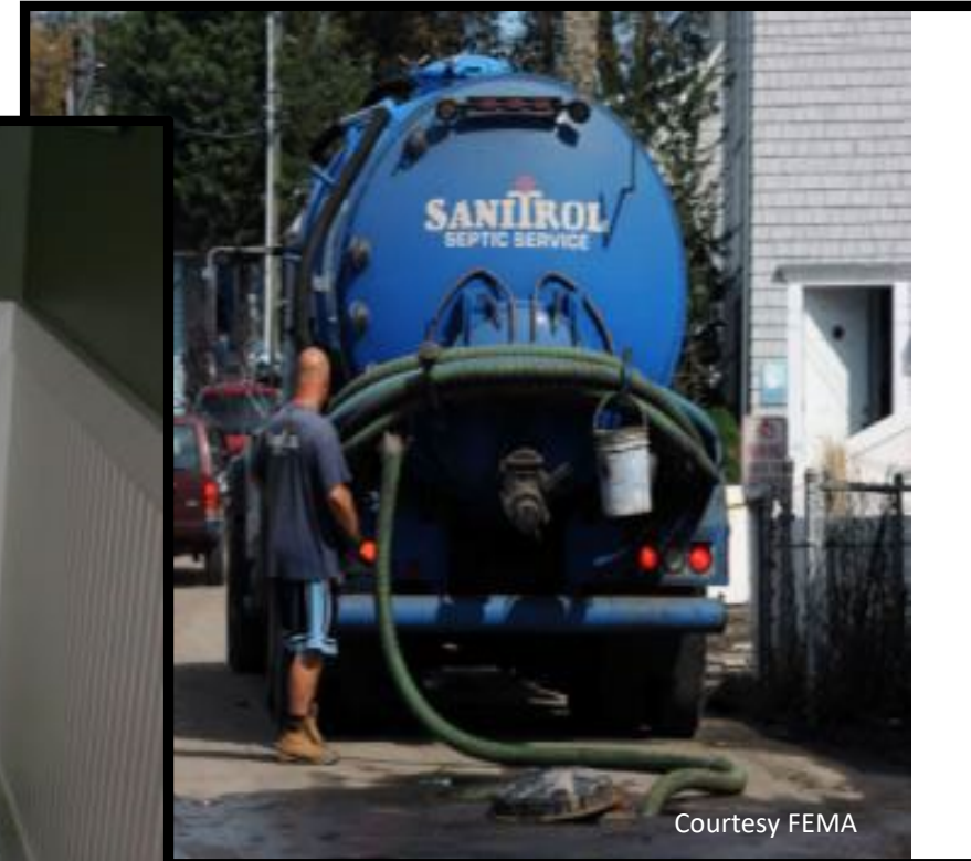
Cleaning up sewage spills or arranging pumping due to power loss at main lift station
