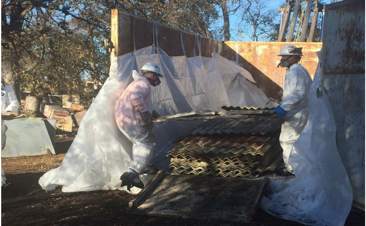
Transite Roofing (Asbestos-Containing Material). (McCourtney/Lobo Fire – Nevada County – 2017)
